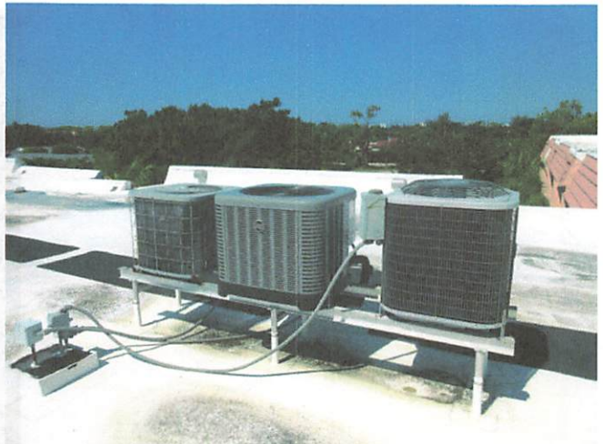
GENERAL VIEW OF HVAC EQUIPMENT
